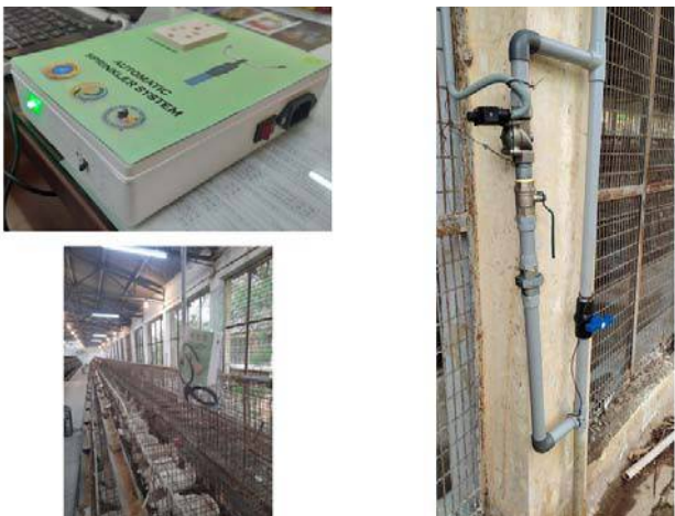
Fig. 8. Automatic sprinkler system installed at DPR, Hyderabad
