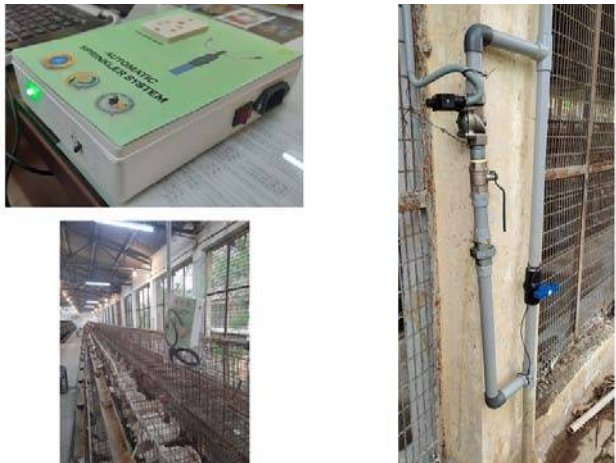
Fig. 8. Automatic sprinkler system installed at DPR, Hyderabad
